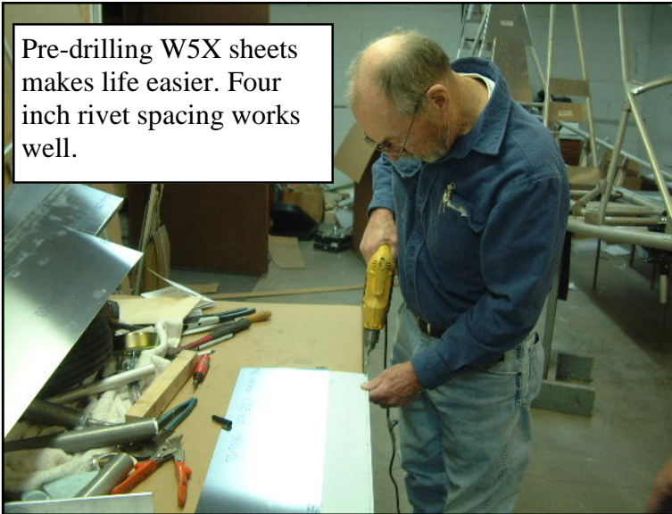
Clecos and clamps make things easier. In-board top W5X sheet being installed.
